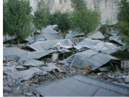
Figure 8: “Collapse of unreinforced concrete block masonry houses in Kamsar near Muzaffarabad,” [7].
